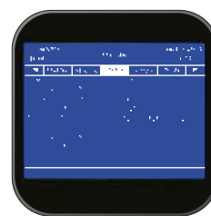
UPS Cabinet Control Panel
